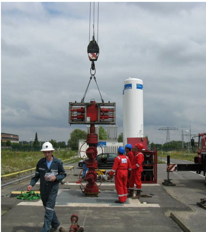
Installations at Ketzin, Germany
